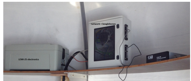
Figure 7. Electronics on a shelf in the radome.
