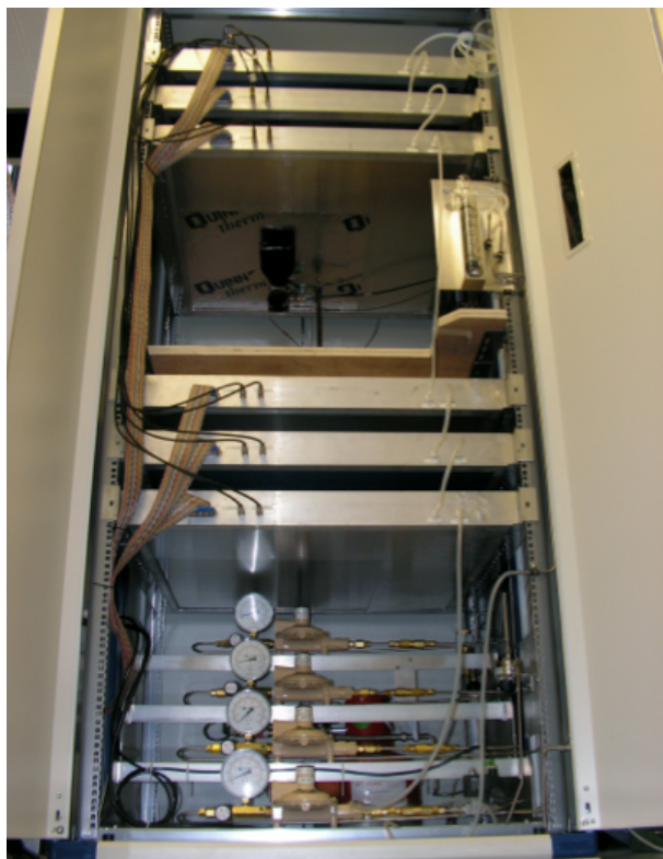
Fig. 2. (Left) picture of the fully assembled system. The six aluminium cassettes contain two RPCs each and provide X - Y readout. The cassettes also provide connections for high voltage, low voltage, data and gas lines. The gas mixing system is visible at the bottom of the cabinet.
