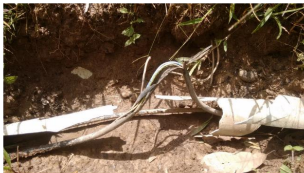
Figure 11. The power cable between the variometer house and the electronics house was damaged a few meters from the variometer house due to currents induced by a lightning strike close to Tatuoca observatory on December 31 st , 2016.
