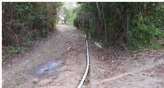
Figure 7. The plastic tube is shown that is used to protect the power supply and fibre optics cable running from the electronics house (visible at the far end in the image) to the variometer house (not visible).
