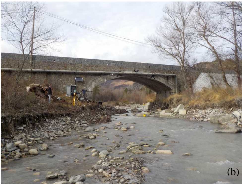
5 Figure 13: Overview (from downstream) of the river section where the RIPLE platform is located on a) the Romanche in Bourg d'Oisans ( 45.1158^{\circ}\text{N} , 6.0134^{\circ}\text{E} , elevation 710 m) and b) the Galabre in La Robine sur Galabre ( 44.1586^{\circ}\text{N} , 6.2360^{\circ}\text{E} , elevation 680 m).
