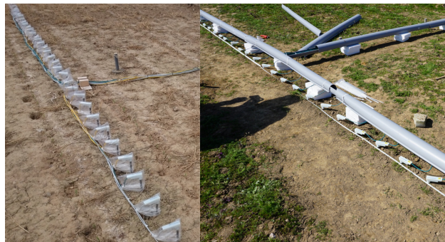
Figure 4. Installation of electrodes, electrode modules, and connecting cables. Left: Installation in 2017, right: Installation in 2018.
