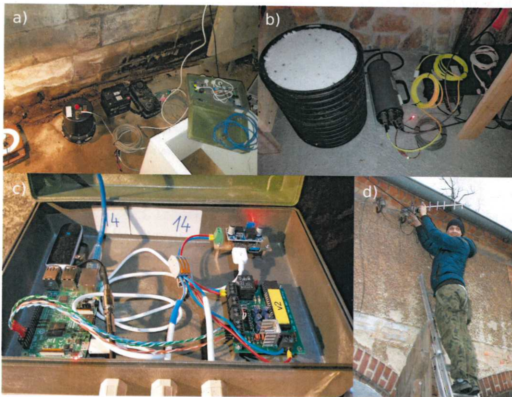
Figure 2: Deployment of seismic stations in Sudetes: a) Reftek unit during installation, b) Installed Guralp unit, c) data-transmission module – Raspberry Pi microcomputer with UMTS modem and watchdog, d) Installing the UMTS antenna for data transmission.
