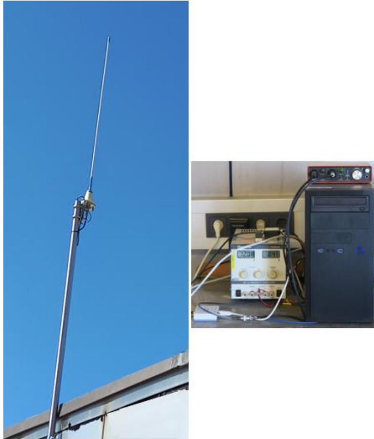
Figure 2. Photo of the new reception system in operation since 2019. The left and right panels display, respectively, the new antenna (i.e., Procom BCL 1-KA) rigidly fixed on a pole and installed on the roof of the building/institute, and the detected radio signal is processed/digitized by a sound card Focusrite Scarlett 2i2 which is connected to a PC running under a Linux operating system. The electronics boxes, power supply, and connecting cables are in an air-conditioned environment. The compact arrangement of devices still enables easy maintainability.
