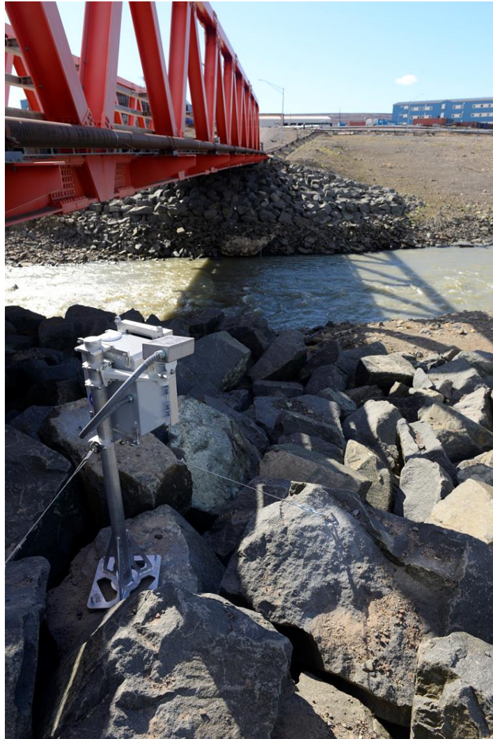
475 Figure 3: Bank-mounted, oblique-looking Laser rangefinder recording river stage on the right bank of the North River, Thule AB. In total, four identical Laser rangefinder units were built and installed in NW Greenland, with two at the Minturn River (Inglefield Land), one at the North River (Thule AB), and one at Fox Canyon River (Thule AB). The single-shot Laser rangefinder measures distance between the sensor and water surface using time-of-flight of the emitted and reflected beam. This novel approach to river stage measurement avoids contact with water, reducing risk of sensor damage or loss from ice, rolling cobbles, and spring breakup 480 floods (photo by Lincoln Pitcher).
