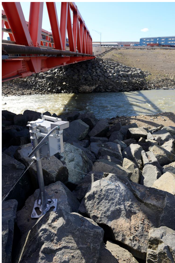
445 Figure 3: Bank-mounted, oblique-looking Laser rangefinder recording river stage on the right bank of the North River, Thule AB. In total, four identical Laser rangefinder units were built and installed in NW Greenland, with two at the Minturn River (Inglefield Land), one at the North River (Thule AB), and one at Fox Canyon River (Thule AB). The single-shot Laser rangefinder measures distance between the sensor and water surface using time-of-flight of the emitted and reflected beam. This novel approach to river stage measurement avoids contact with water, reducing risk of sensor damage or loss from ice, rolling cobbles, and spring breakup floods (photo by Lincoln Pitcher).
